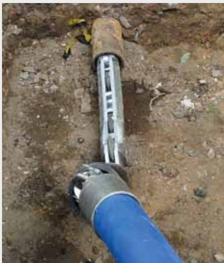
Sao Paulo: The new roller cutter cuts a ductile cast iron pipe 5" first in Brazil.
