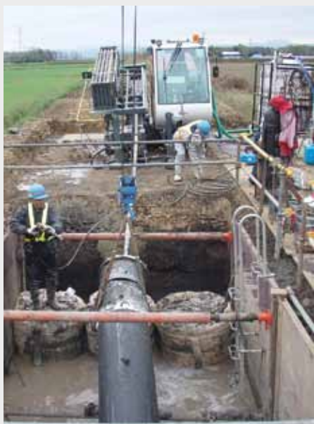
Japan: The TERRA-JET 8522 S lays a HDPE pipe OD 560 mm (22") over 60 m (200 ft).
