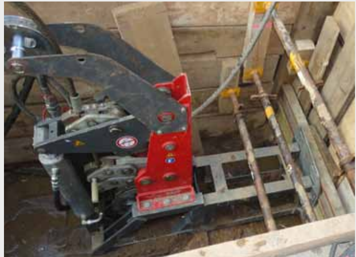
Düsseldorf: The cable burster X 400 replaces an old cast iron pipe over 60 m (200 ft) and pulls in a new HDPE pipe OD 110 mm (4.3").
