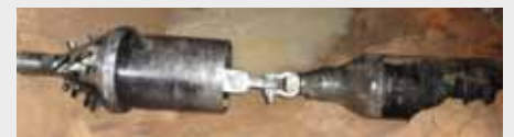
Turkmenistan: The backreamer Ø 420 mm (16.5") and the steel pipe Ø 300 mm (12") reach the target pit.
