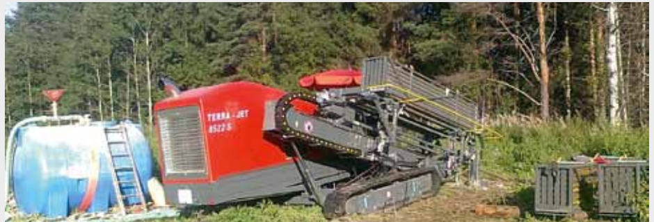
Russia: The company Reljef during their longest HDD bore. Die pilot bore runs over 324 m (1'070 ft) under the forest. A HDPE pipe OD 225 mm (9") is pulled in.
