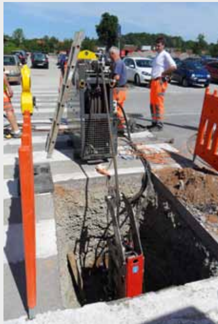
Crailsheim: The automatic cable drum X 400 rolls up the pulling cable simultaneously to the pipe pulling.
