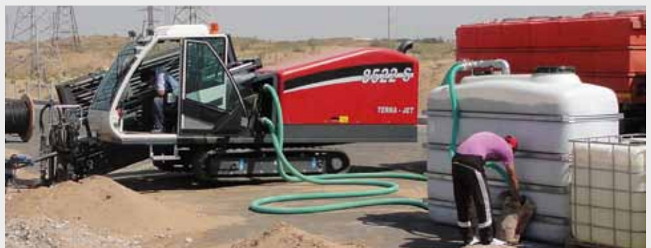
Turkmenistan: The TERRA-JET 8522 S Premium during the pipe pulling. Just now Bentonit is mixed in.
